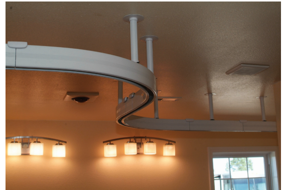
A lift system runs from the Master Bedroom to the Master Bath
